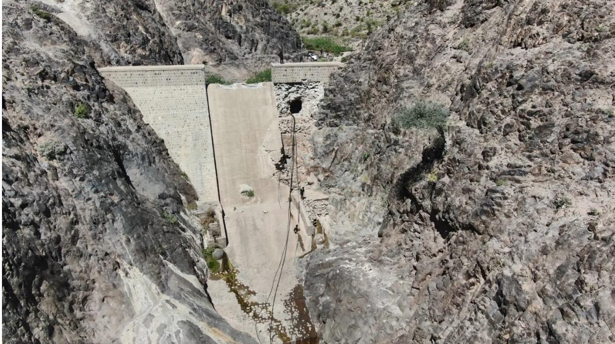
An aerial drone image showing the gate of Al-Nukhila Dam in Al-Azariq after being damaged as is visible in the photo, Jan. 2024 ('South24 Center')
